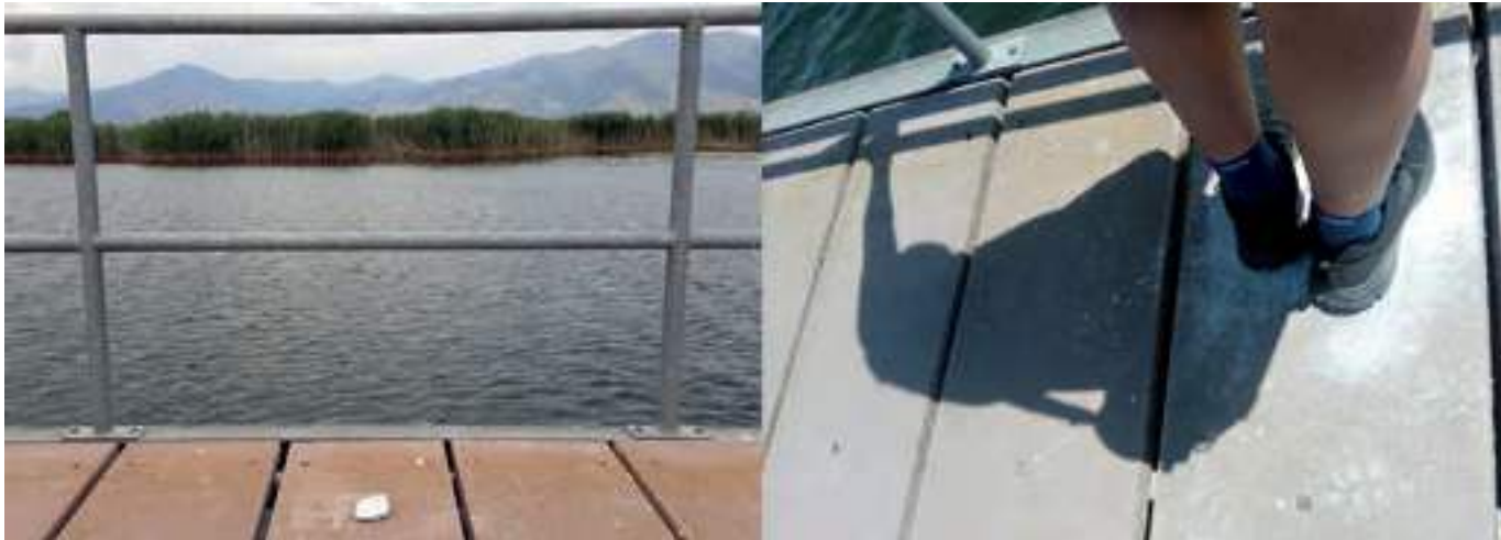
Figure 4. Incidental Path: Crushing the Stucco (Agios Achilleios pontoon bridge)
