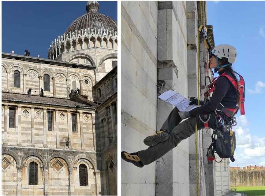
Fig. 1-2 The conservator is mapping critical areas on the architectural survey while suspended by ropes.
